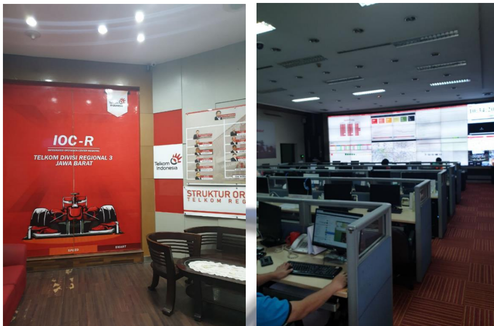
Gambar III - 4 Ruang ROC Regional 3
